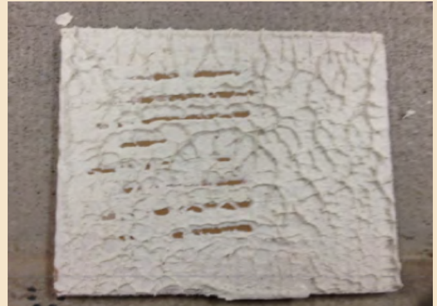
6" x 6" (150mm x 150mm) quarry tile installed using a 1/4" x 1/4" (6mm x 6mm) square notch trowel – sufficient coverage has been achieved.
