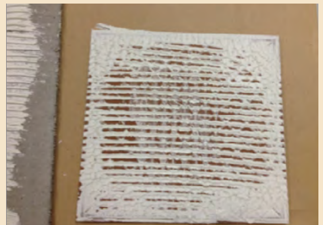
18" x 18" (450mm x 450mm) tile installed using a 1/4" x 1/4" (6mm x 6mm) square notch trowel – insufficient coverage has been achieved.
